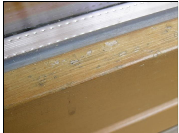
Fig. 3.1: Hail damage to the window
